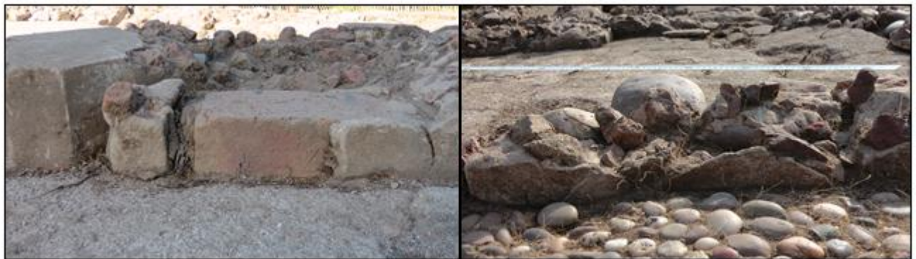
Plate 11 Depicting the variety of building materials used in the construction of the buildings
